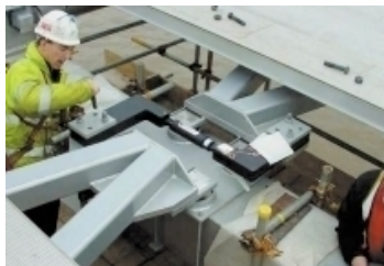
Figure 1. Installation of viscous dampers beneath the deck of the London Millennium Bridge
