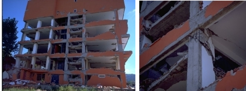
Figure 1. Damaged RC frame with hollow clay tile infill masonry, Izmit 1999 (Elwood et al. , 2000)
