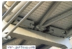
Figure 2. Tuned mass dampers beneath the deck of the London Millennium Bridge
